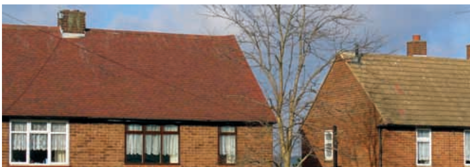
Left: Both of these properties were roofed in the 1960's, with red roof tiles. The house on the left of the picture was tiled in Dreadnought Red clay smoothfaced tiles; the house on the right with Red concrete tiles. The picture taken 40 years later shows that whilst the clay roof has remained a rich red colour, the concrete roof has faded to a grey colour, and lost all its pigmentation.
