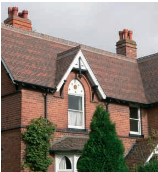
Above: Re-roofing of Victorian House using a mixture of Brown Brindle and Country Brown Tiles with Ornamental Club Tiles to match the original. Ornamental finials and ridge tiles were hand-made to match the original.
