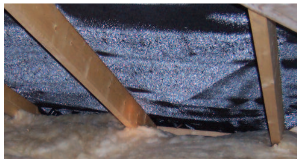
Impermeable underlay (type HR) with flocked underside showing condensate being held.
